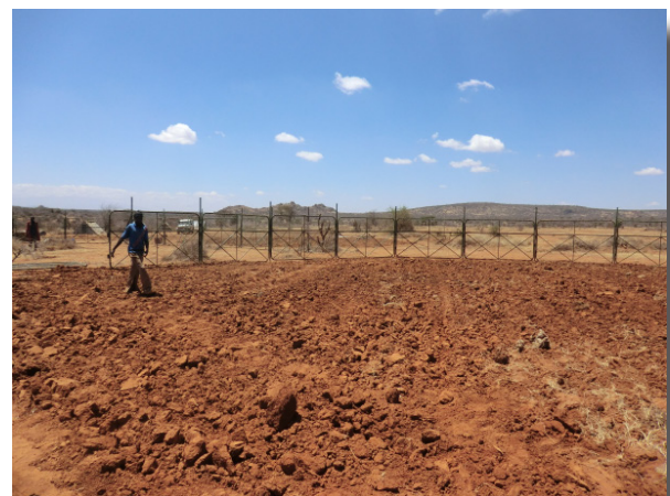
Tractor ripping before the cattle boma is placed on site. All photos by David Kimiti.
